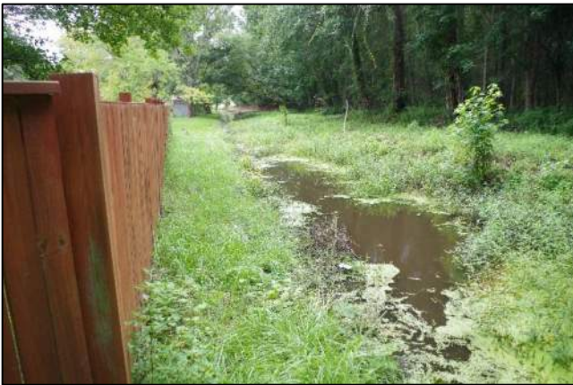
Photo 27. Ditch Full and Overgrown 8/25/17
