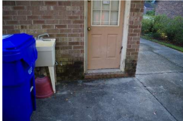
Photo 7. Finished Floor above Ground Surface
