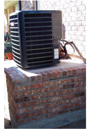
Raise outdoor equipment above your flood level
