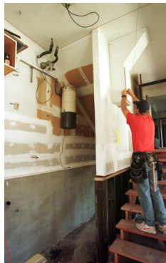
Moving a water heater above ground level will help save the appliance and keep it working during a flood. Photo by: Dave Galley/ FEMA
