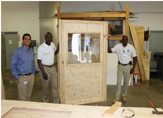
Charleston County Facilities building testing booths.
